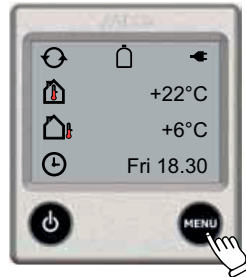
Control panel in standby
